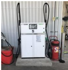
Station distribution gasoil et sans plomb
